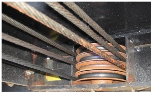
Rust on sheave stack and ropes
